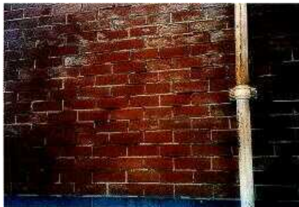
Failed pointing – open joints.
