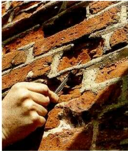
Detached hard pointing.
