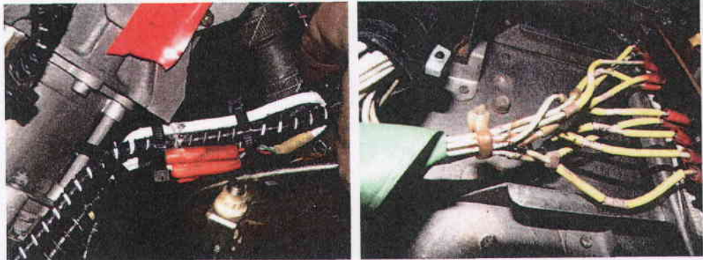
Figure B-7; damage to electrical cables
