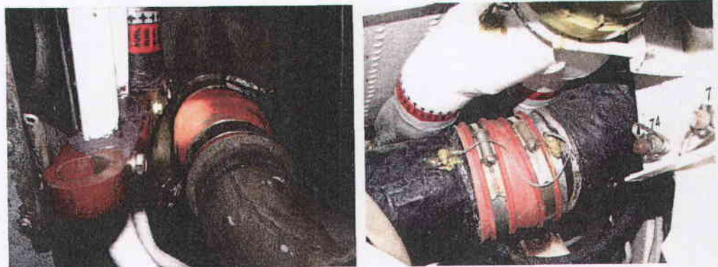
Figure D-6; Insufficient clearance between ducts and fuel pipes
