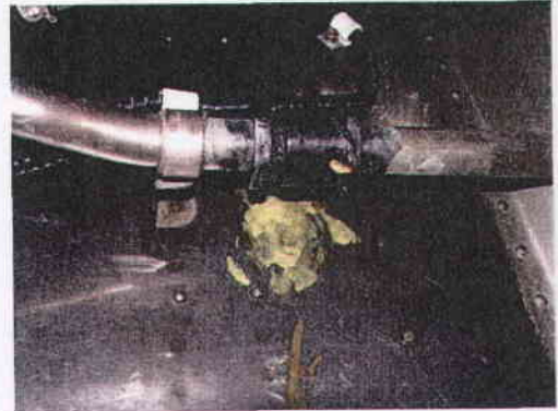
Figure D-16; Signs of overheating of protective coating
