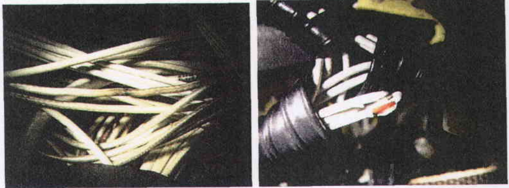
Figure D-13; Damage found on electrical cables
