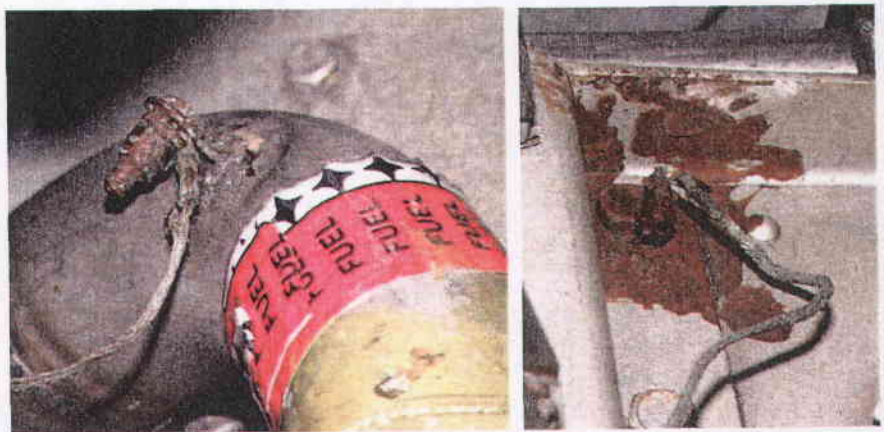
Figure D-14; Damage found on bonding leads
