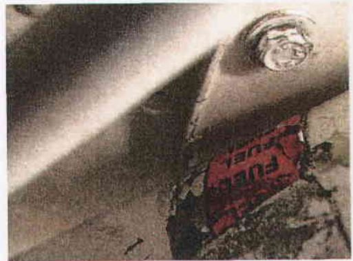
Figure B-2; A2, Chafing, Zones 133/134, No 5 tank Cell 2 pipe chafe apparent from panel ridge trim
